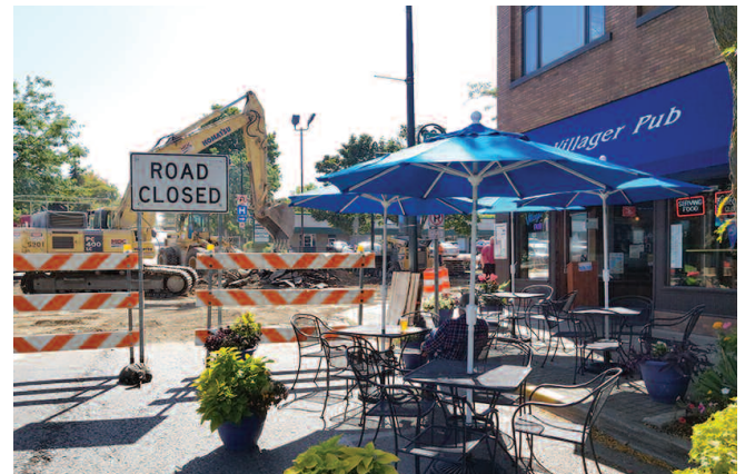
Business as usual despite the road closing, including the Farmers market on Bridge street 8am to 1pm Thursday. Just turn on Mason, you may still park on Bridge Street. The construction is projected to be done in two weeks. PHOTO BY M. CHRIS LEESE.
